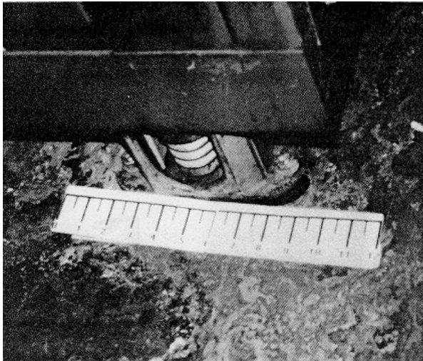
Figure B-7. Vulnerable engine generator vibration isolation system
