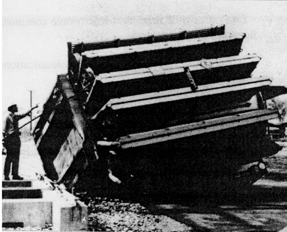
Figure B-2. Failure of a rail-mounted transformer
